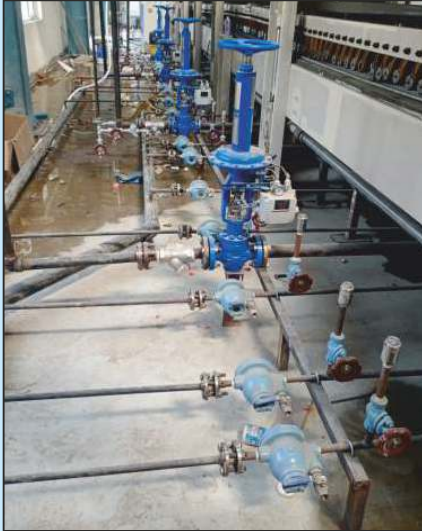
INSTALLATION OF CONTROL VALVE & TRAPS ON PACKAGING MACHINE
