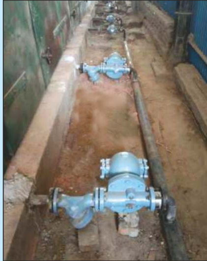
FLOAT TRAP INSTALLATION DRYING MACHINE IN PLYWOOD INDUSTRY
